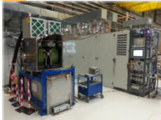
FOS debuncher cavity SAT ongoing.
