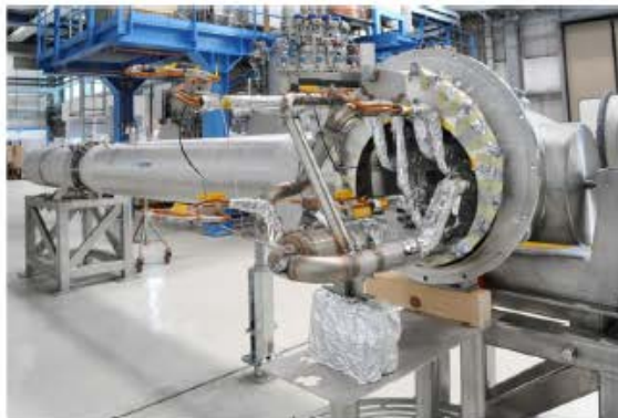
First cryogenic bypass line delivered and under cold testing at GSI (Poland)
